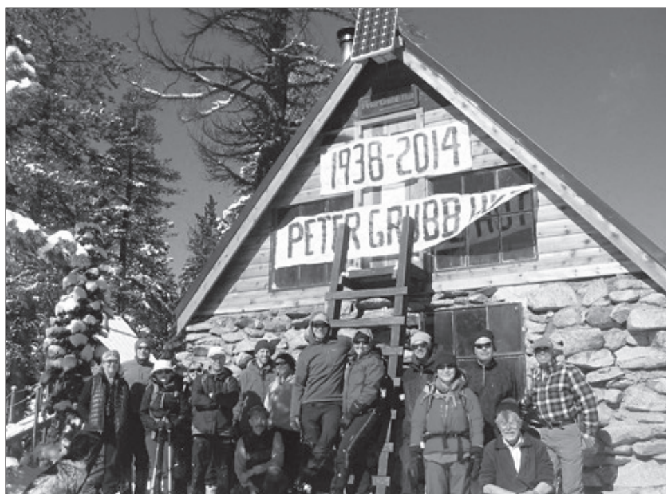
Volunteers at the Peter Grubb Hut as structural repairs neared completion in November 2014.
