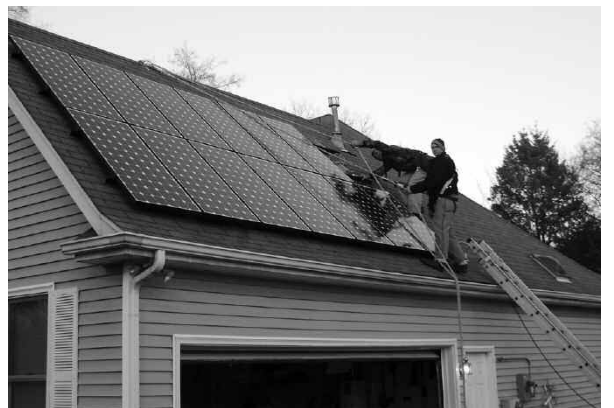
This 3.15 kW solar PV installation in Rockvale, Tenn., near Murfreesboro was one of the first homes to take advantage of the 30% tax credit without the $2,000 cap. Photo courtesy of LightWave Solar Electric.
