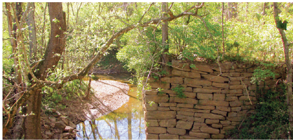
A bridge abutment built by US soldiers in 1801 by order of President Thomas Jefferson for the wooden bridge that crossed over Brown's Creek by the Harpeth River at Old Town. Photo by Marsha Comstock.
