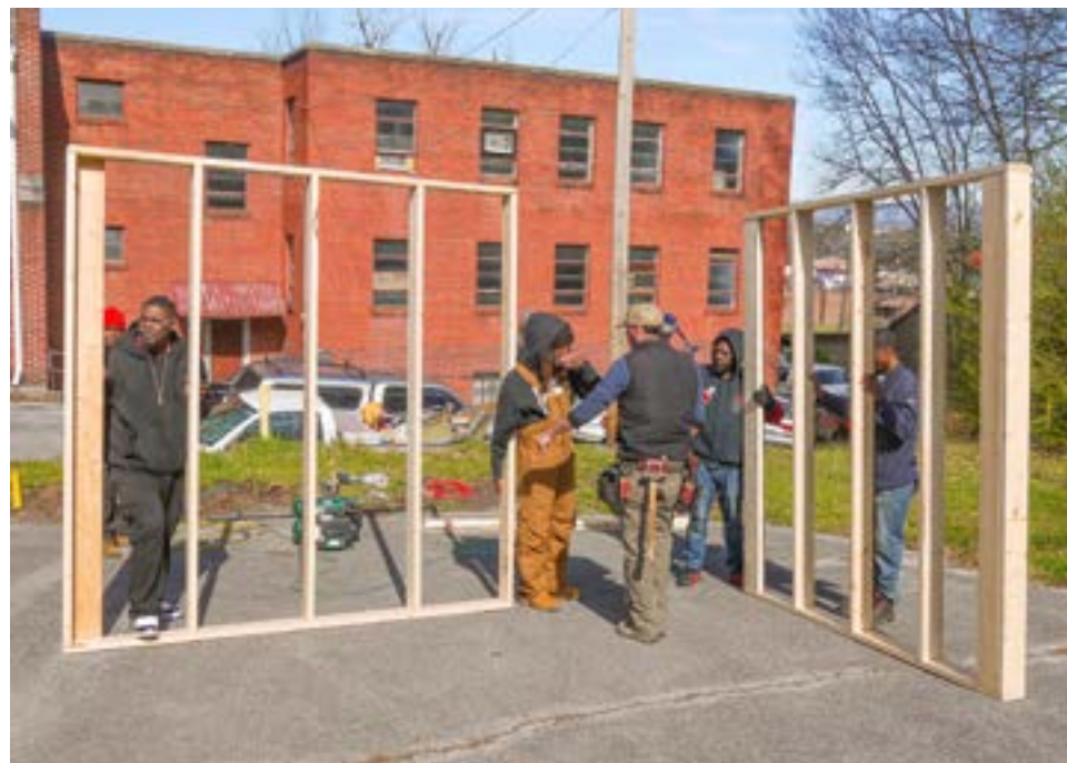
Above: Build It Green participants learn advanced framing techniques from professionals at New Blue Construction.
