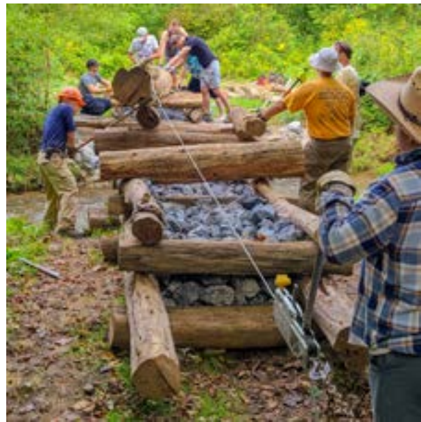
Volunteers building Jacob's Bridge over Sinking Creek in Jacob's Nature Park, Johnson City, Tennessee.
