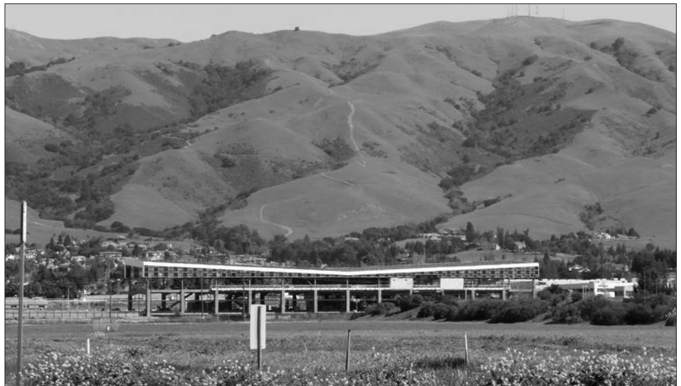
Warm Springs BART station under construction in background; development with 2,200+ houses planned for area in foreground.
