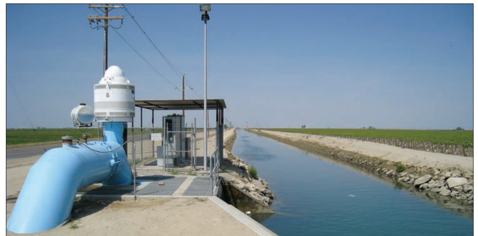
Canal and tank of the Semitropic Water Bank. Photo courtesy Chris Austin on Flickr.
