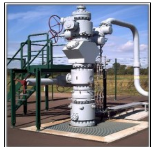
Deep injection wellhead/Photo from FDEP
