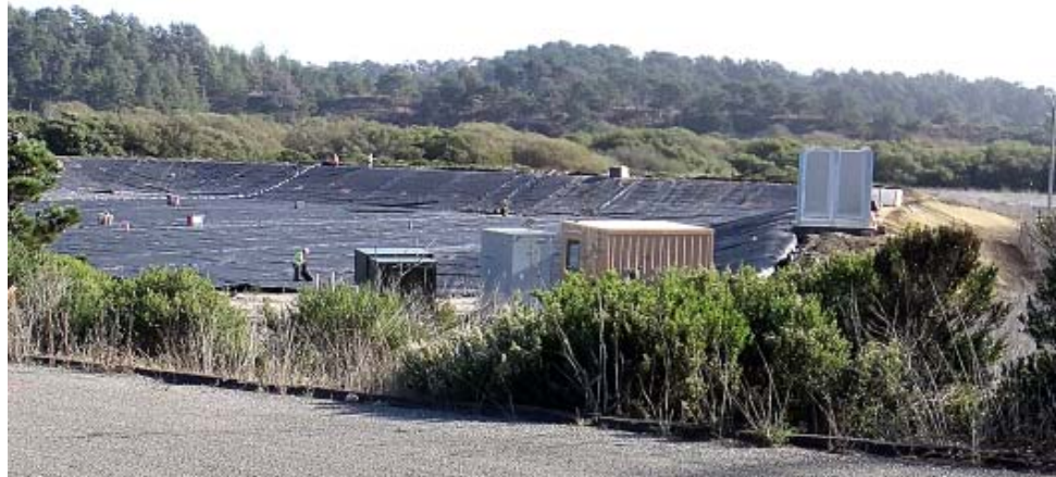
The perils of cutting corners The Cambria CSD's malfunctioning desal brine pit is just one of the chickens coming home to roost in the attempt to parlay a fake emergency into a water source for future development.
