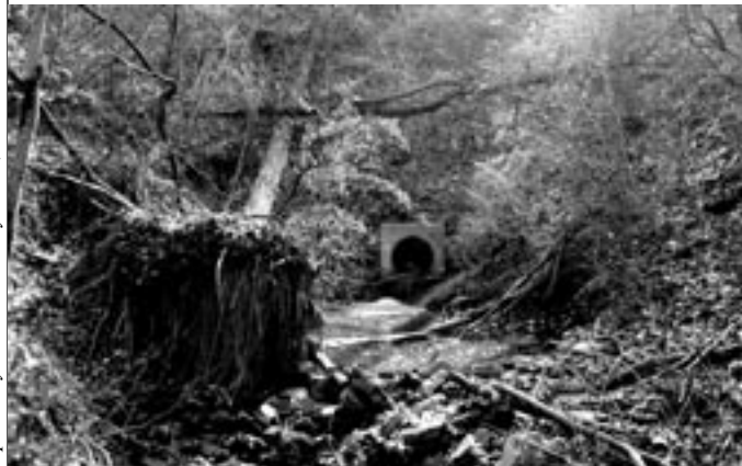
Exposed storm drain at the end of Texas Avenue, N.W.
