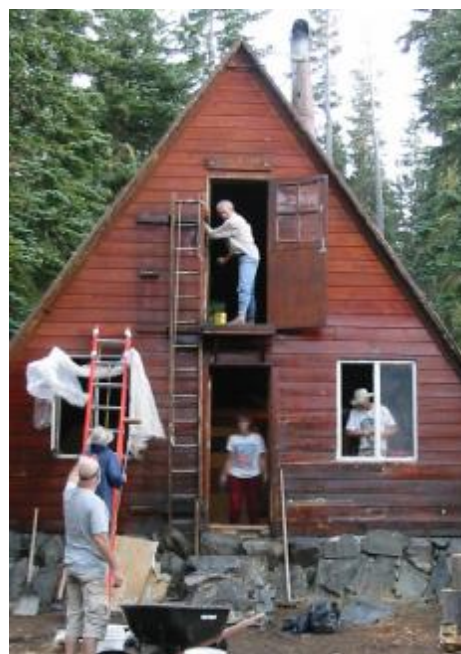
Staining and window repair at the front of the hut; John Ebneter (left), Jim McPherson, Tony Stieber (upper landing), Hella Stieber, and Bob Creek (right).
