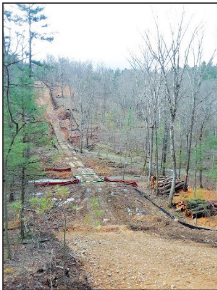
Slope erosion is a problem at the Kesecker Farm in Morgan County.
