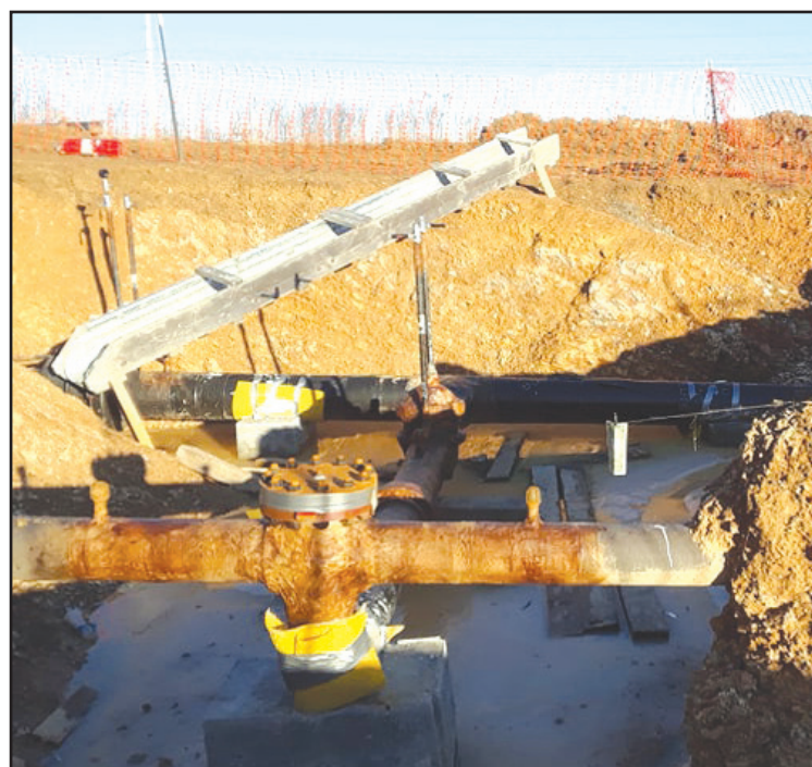
The only gas source in the Eastern Panhandle at this time is the 6-inch Washington Gas Light line in Clearbrook, VA, a pipeline that is about 60 years old and already running at its maximum allowable pressure. The dollar bill hanging above the pipeline establishes scale.
