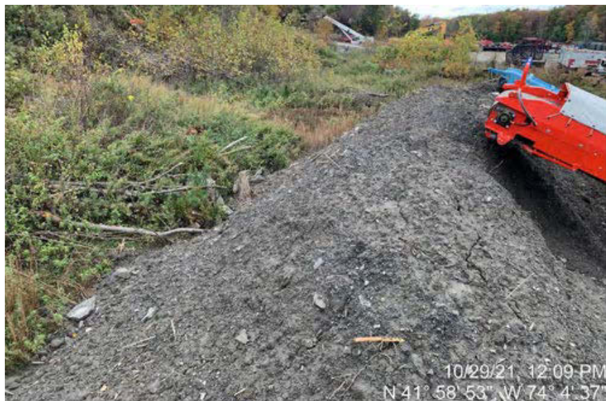
Photo 12: Material Stockpiles with no erosion controls.
