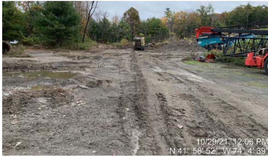
Photo 11: Disturbance along eastern side of pickerel pond.
