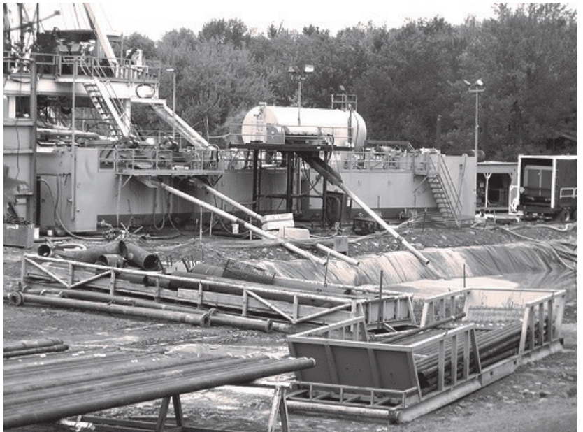
This photo shows drilling muds pouring out of the drill rig into lined pits.
