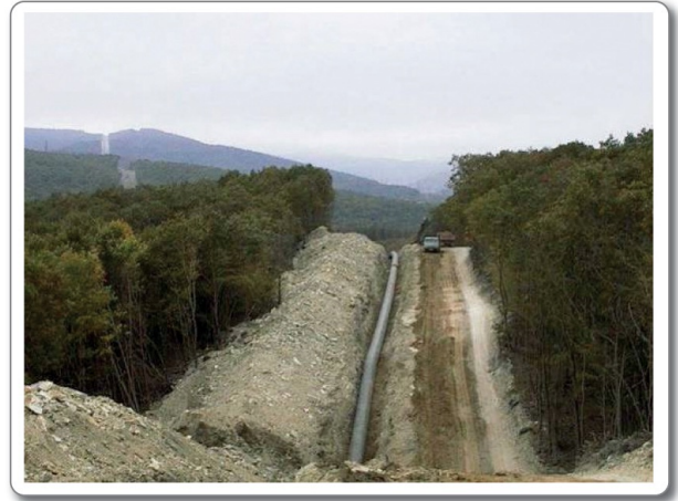
A gas pipeline running through New England
