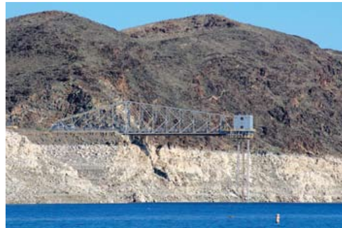
Las Vegas water intake at Lake Mead seen in 2009. Photo: D. Ghiglieri.
