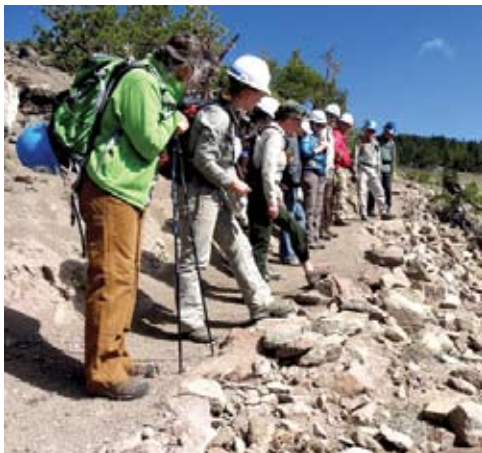
Building the Houghton Spur at Relay Peak, summer of 2014. Photo: Tahoe Rim Trail Association.
