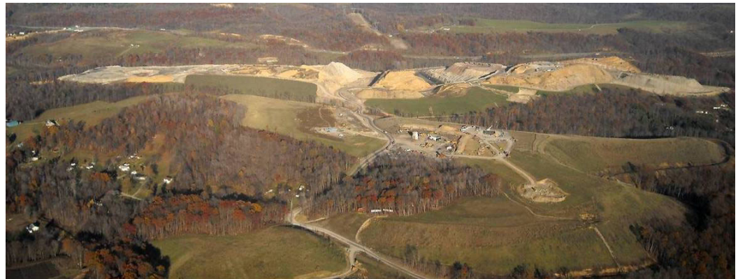
Mine complex about 3 miles in length visible from I-79 just north of Morgantown. Part of New Hill West permit area is in the lower left of this photo.
