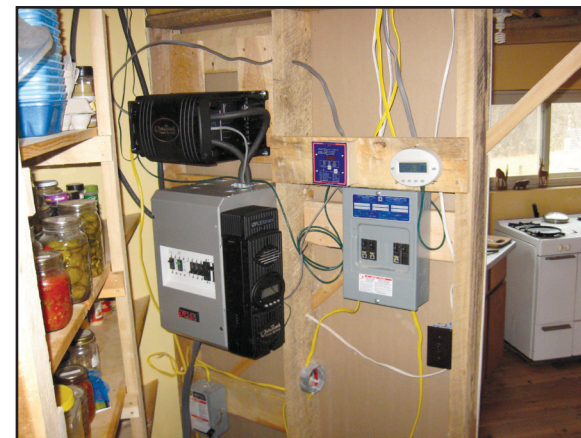
The electronics — inverter, charge controller and meters — for an off-grid system are accessible from inside the house.
