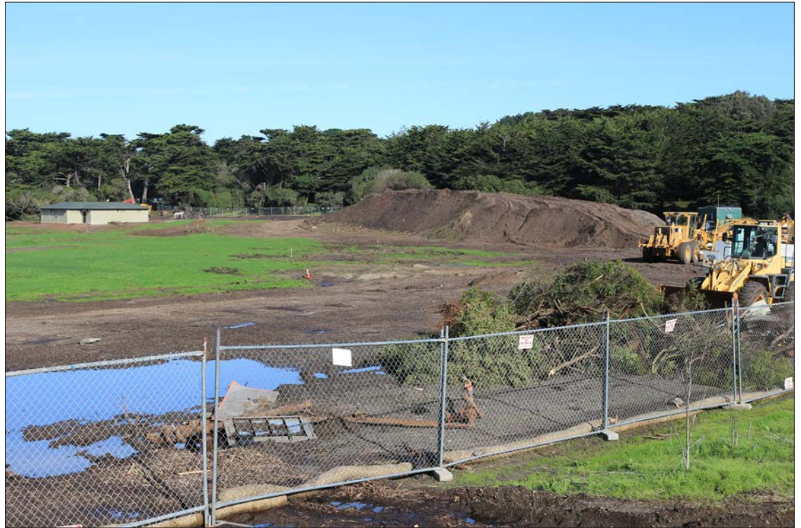
Construction on the Beach Chalet soccer fields as of January, 2015. Photo by Kathy Howard.
