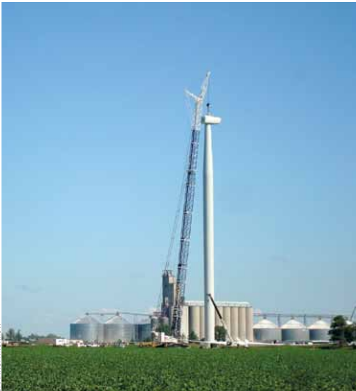
This wind turbine is part of Michigan's 30,000-acre wind farm in northeast Gratiot County.
