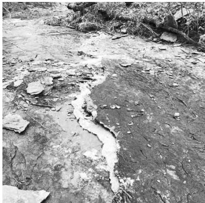
A crack in the stream bed that has led to the emptying of the water
