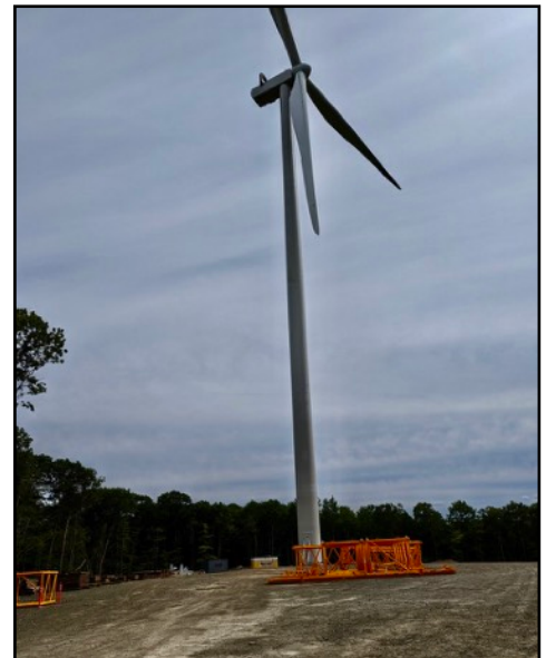
Newly-installed, not yet operational turbine, Town of Windsor. photo Scott Lauffer
