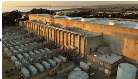
1.6 GWh at Moss Landing, California 2021
