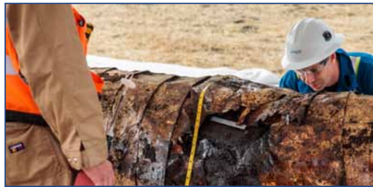
Trouble spot: The notorious oil leak from Plains Pipeline Gaviota Coast, due to poor maintenance and delay in stopping it because it did not have an automatic shutdown. Oil spilled into the ocean, closing beaches, harming animals, sparking lawsuits, and adding to anti-oil sentiments. Photo by Bruce Reitherman - Santa Barbara County, 2015
