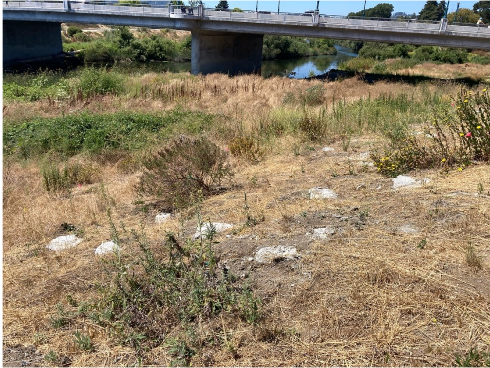
Grout covering non-rodent depressions as well as rodent tunnels
