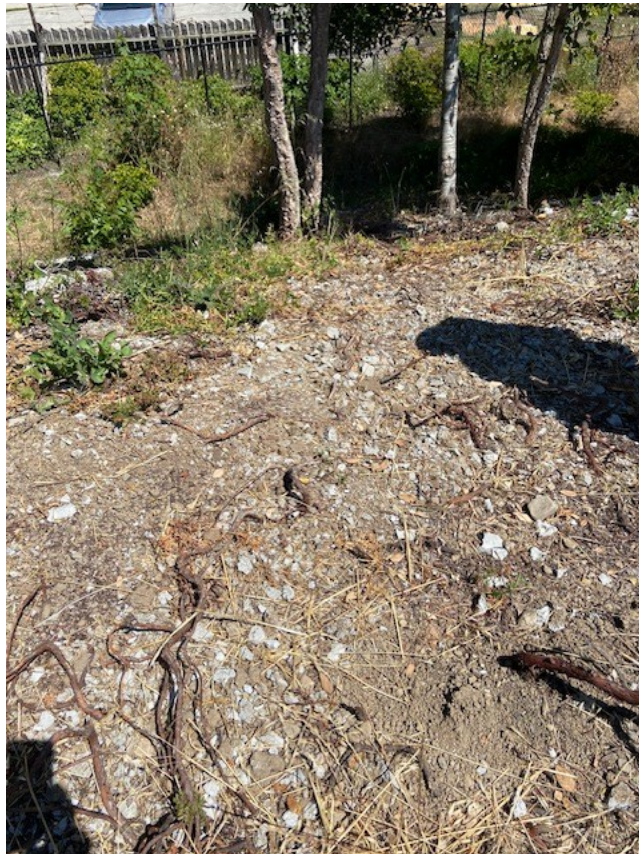
Excessive grout debris spread during application
