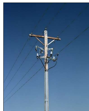
Transmission lines. Photo By: Warren Gretz, National Renewable Energy Laboratory
