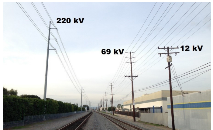
EXISTING ANAHEIM PUBLIC UTILITIES TRANSMISSION AND DISTRIBUTION LINES, WITH VOLTAGES SHOWN, SHARING A SECTION OF THE 100'-WIDE LOS ANGELES- SAN DIEGO AMTRAK PACIFIC SURFLINER LOSSAN DOUBLE-TRACK RAIL CORRIDOR (PHOTO BY BRIAN YANITY)
