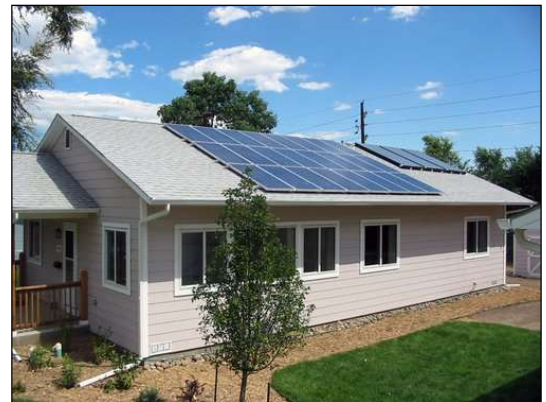
Solar panels on rooftop. Photo Credit: National Renewable Energy Laboratory
