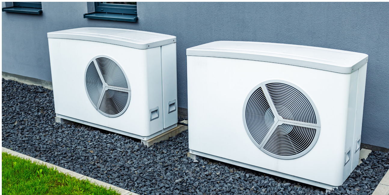
Air-Source Heat Pumps
