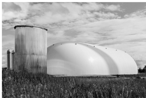
CO2 battery facility in Sardinia, Italy
