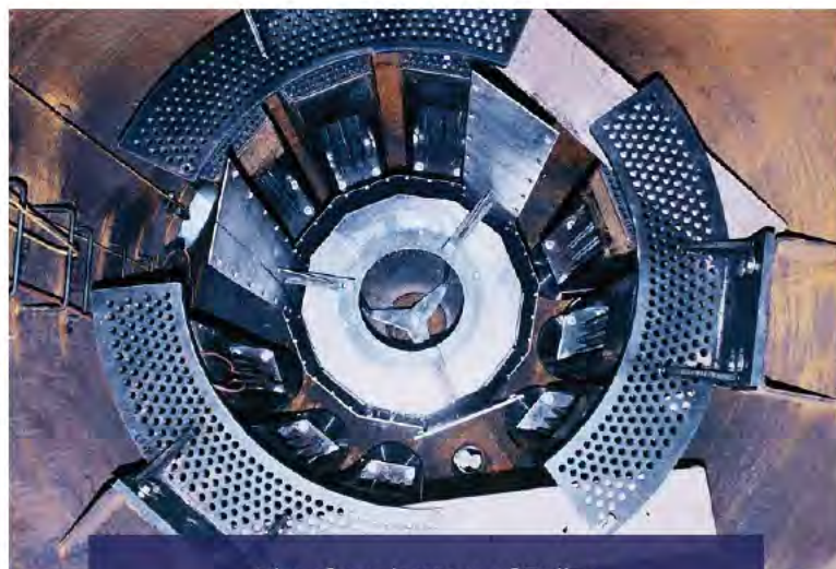
View from bottom of Boiler with 9 Electrode Boxes
