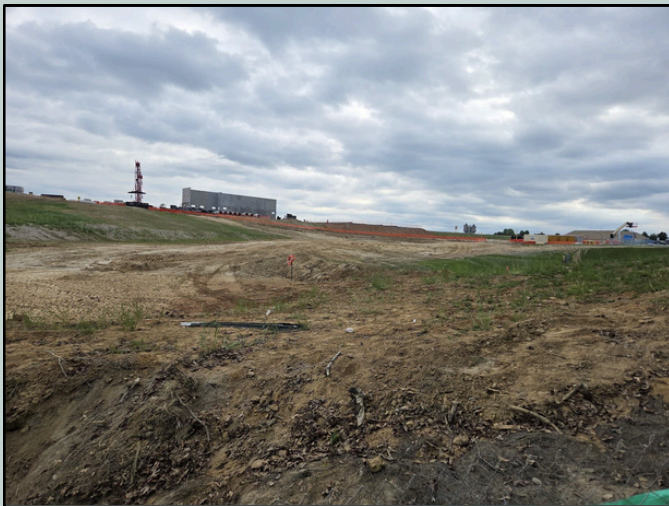
April 26th First wall of STC put up off of Richmond Highway, photo taken uphill from Stream 1, which flows through the middle of the property
