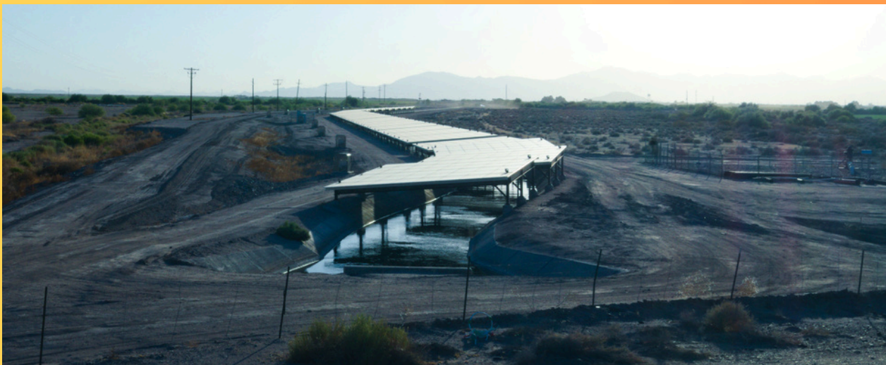
Gila River Indian Community Solar Canal Project. Photo by Miché Lozano
