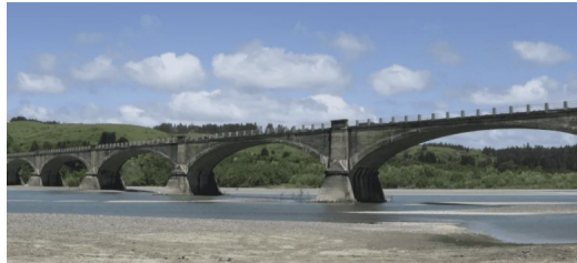
The concrete arch Fernbridge is the first bridge to span the Eel above its mouth. (Photo/Public domain)
