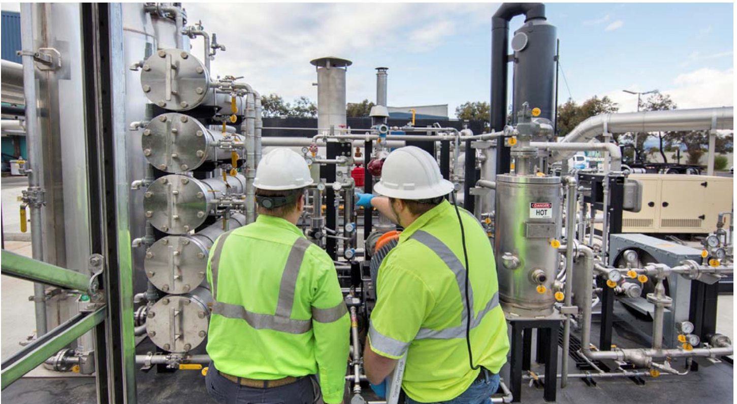
Workers inspect an anaerobic digestion solid waste processing facility that converts food and green organic waste into biogas.
