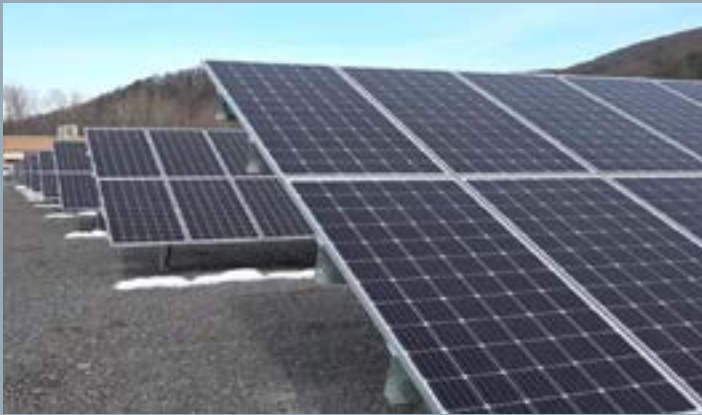
SOLAR PANELS INSTALLED AT THE PETERSBURG ELEMENTARY SCHOOL IMAGE CREDIT: GRANT COUNTY SCHOOLS
