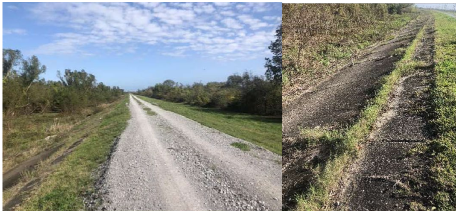
Figure 35a. Crest of river levee fronting LNG site and 27b. river side shown crack concrete capping.
