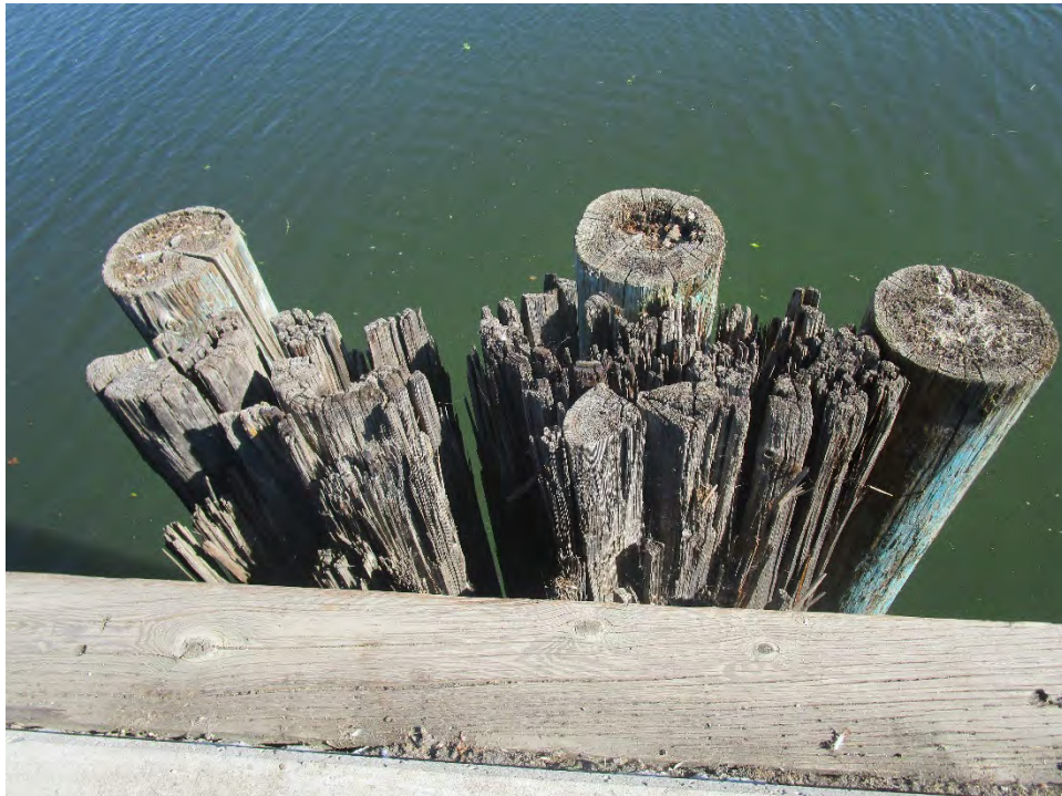
Wooden support piles at the northeast corner of Berth 2; View: Detail; Date: 09/26/19; Acc. #: 19-0016-2302
