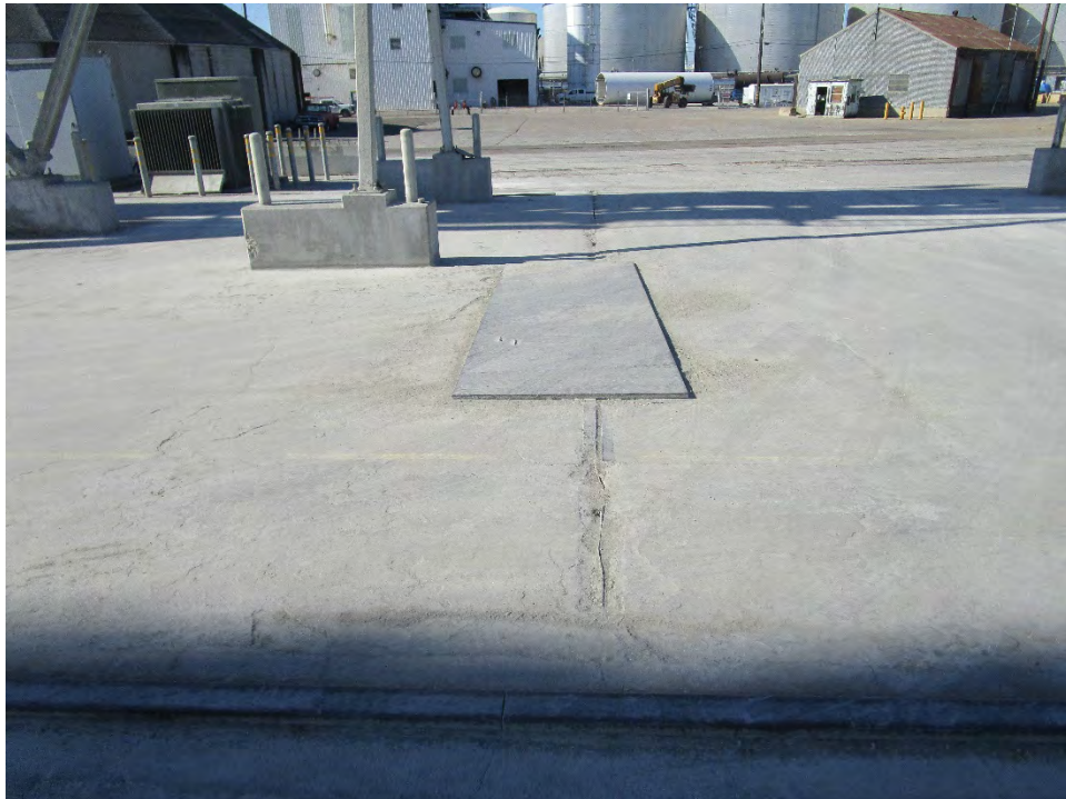
Metal plate covering a sink-hole in Berth 2; View: West; Date: 09/26/19; Acc. #: 19-0016-2300
