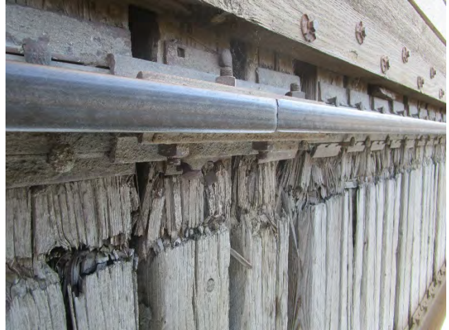
Shearing damage along the western side of the trestle rail; View; North; Date 09/26/19; Acc. #: 19-0016-2295
