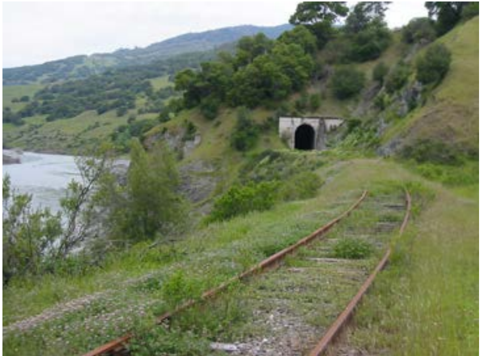
Railroad tracks along the Eel River lie on geologically unstable ground. Some of the tracks have been covered by landslides or have been overtaken by water.
