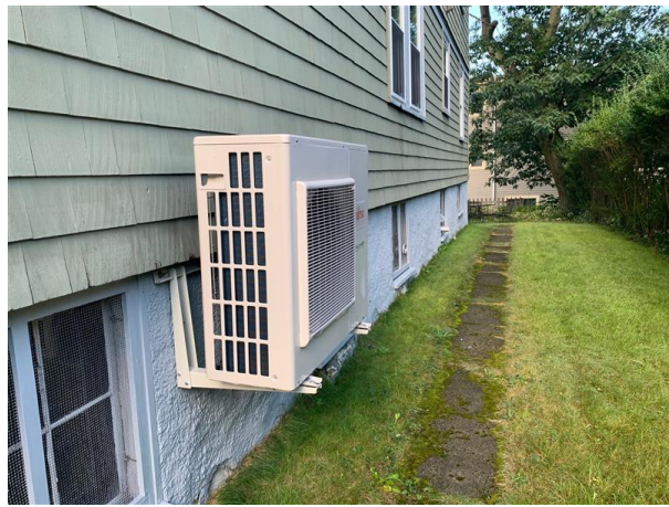
One of the outdoor units for the whole-home heat pump system at the author's home. Meg Howard, Program Director, MassCEC
