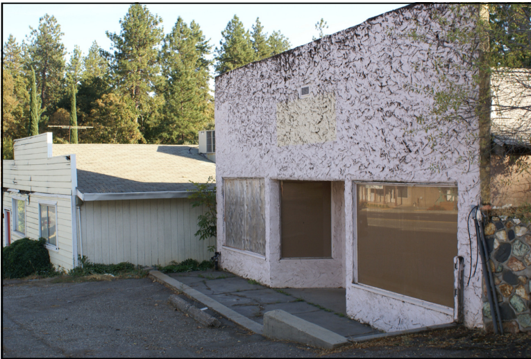
Several empty buildings dot the Skyway Commercial District, some like this are in physical decay. Coming of Wal-Mart may compound the problem of blight.
