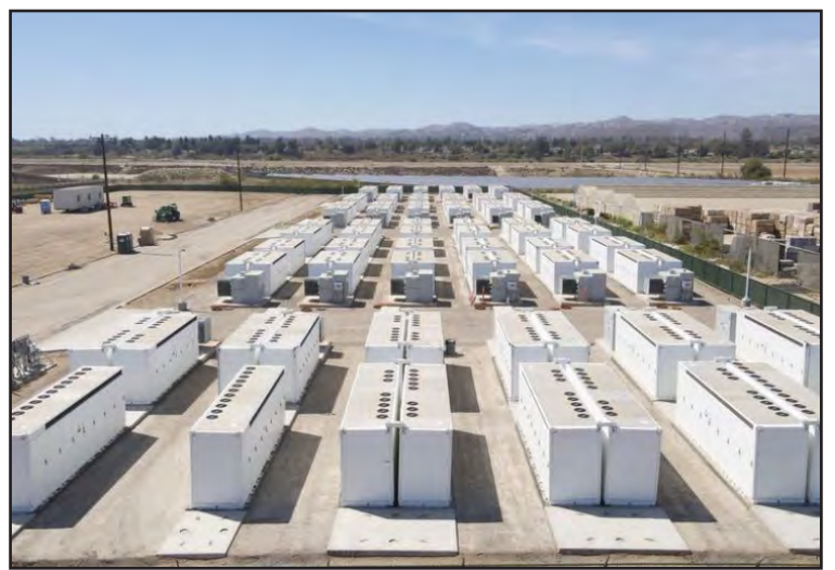
The Salicoy battery energy storage system by Arevon uses 142 Megapacks from Tesla to generate 100mw. This replaces a gas-fired peaker plant initially advocated by SoCal Edison but stopped by activists who wanted cleaner energy. (Arevon Asset Management.)
