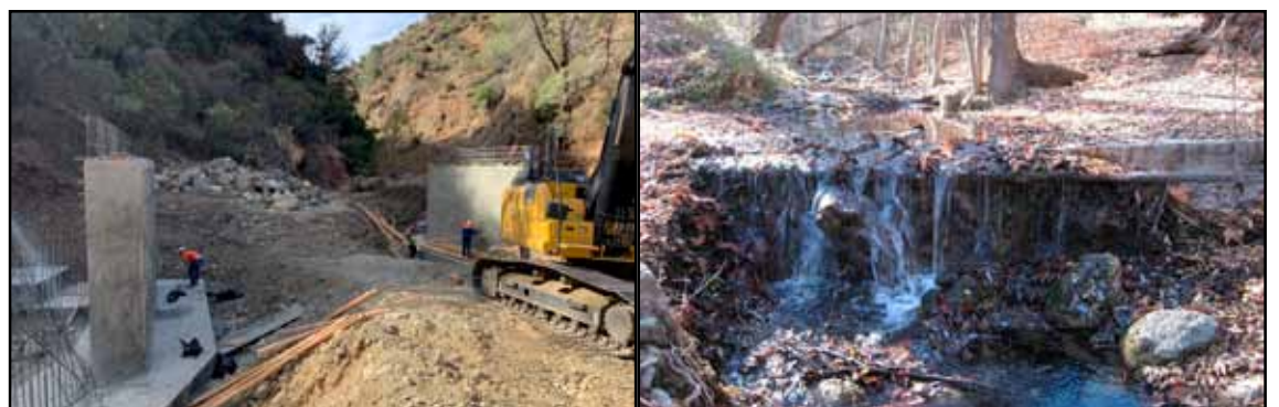
Sunset Valley Road has reopened after an 8-month closure along with the popular Davy Brown and Nira Campgrounds and driving access to a stunning network of trails and opening over three miles of steelhead habitat. Here's one of two bridges under construction (left) and now finished. At right, the Munch Creek Crossing will remain in a natural state with the removal of the low-water concrete crossing. (Photo courtesy LPNF)
