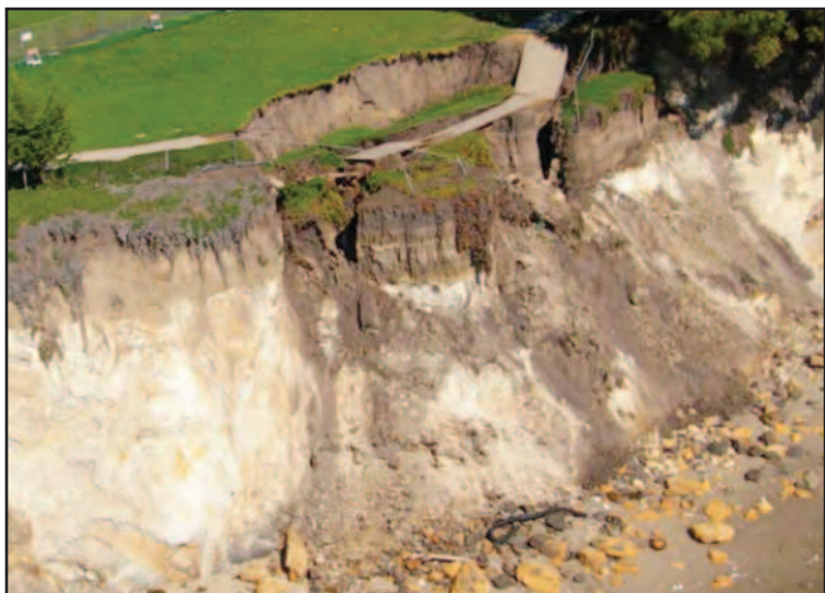
The January 2008 landslide along the cliff at Shoreline Park moved the cliff edge landward by as much as 38 feet and eliminated a portion of the sidewalk. According to Katie Davis, "the ocean is 8 inches higher than it was a century ago and sea level rise is accelerating so cliff erosion will increase. Sea level could rise five feet this century and Shoreline Park could be eroded by 270 feet." (Photo contributed)
