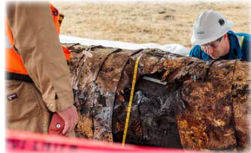
The culprit, a pipeline portion that was seriously eroded and not caught by owner Plains Pipeline. Although a critical portion that connects with the offshore platforms, it was the only pipeline in Santa Barbara County that did not have an automatic shutoff feature. (Photo courtesy of SB Planning Dept.)
