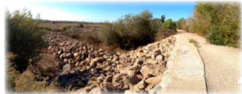
About 17 years ago across the Santa Clara River north bank the county used open rock and vegetated groins for erosion control, and guess what? The groins are doing exactly what they are supposed to do: provide bank stabilization and prevent erosion. (Photo by Nina Danza)
