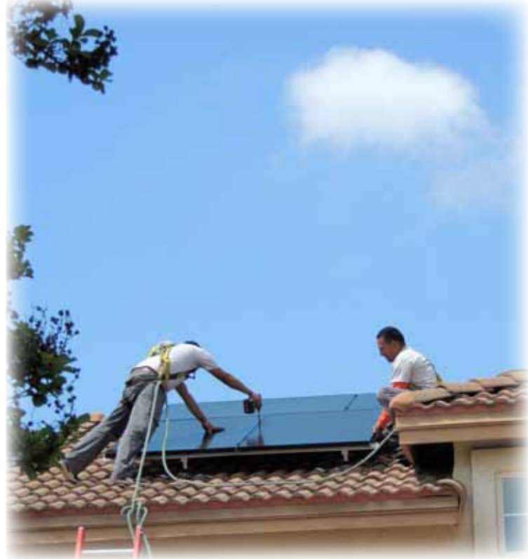
Sierra Club gives discounts to top off your roof with solar panels for cleaner energy; helps our chapter too. (Photo by Condor John)
