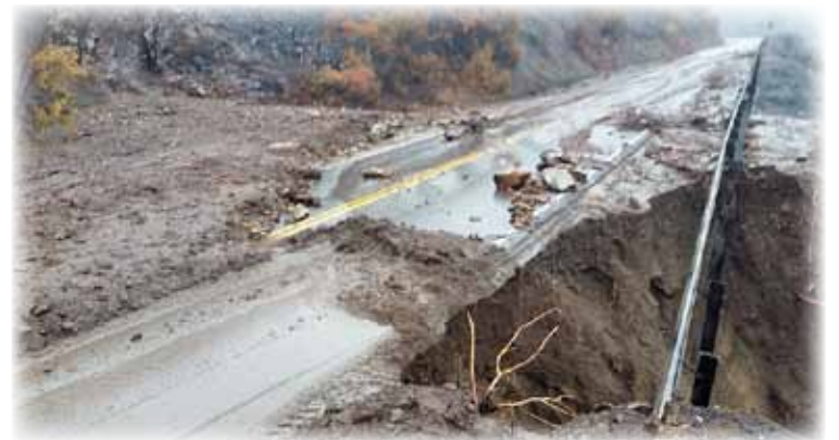
Hwy 33 is closed above Wheeler Gorge due to road damage from the January floods (Photo by CalTrans)
