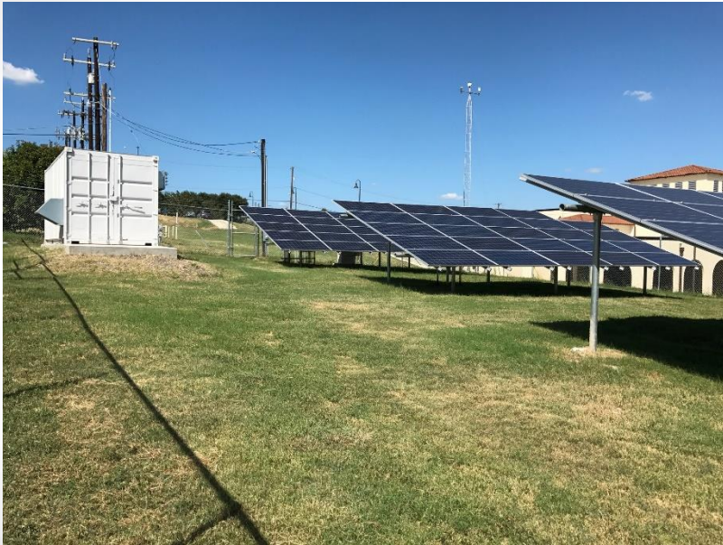
Photovoltaic system paired with a 75kW battery system
